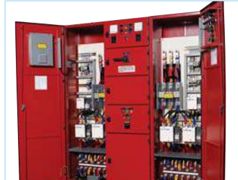
Sprinkler & Hosereel Pump Control Panel
