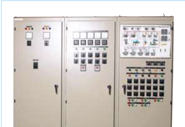
Coolroom Plant Control Panel
