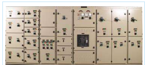
Chiller Control Panel/Main Air Conditioning Switchboard
