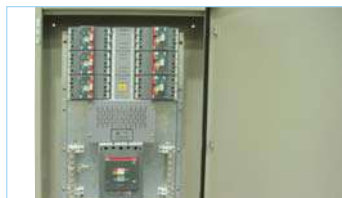
MCCB Pan Assembly Panel Board
