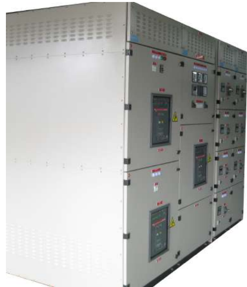
3.1.2.2 Sunlight's Series Forti LV System is designed and tested in 2-tier ACB arrangements
