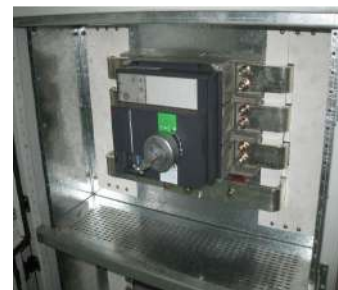
3.1.1.1 The compartment, partition and doors have to withstand the stresses during short circuit conditions
