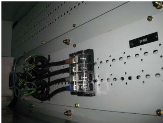
3.1.1.9a Terminal blocks are provided for external cables. Cable support provisions is catered for on the partition plate to secure the external cables
