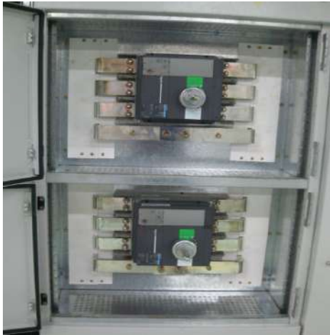
3.2.2a Each functional device i.e. breaker in Series Forti LV System is compartmentalized i.e. Form 3 and
