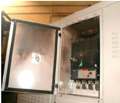
4.7a An outgoing breaker had undergone a conditional short-circuit
