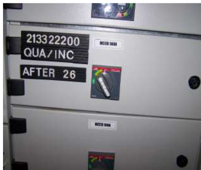
4.7b After short-circuit, the protective breaker must trip, its metal door cover must remain closed and IP be maintained
