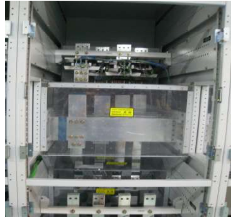
3.1.1.6 Barriers are provided to protect personnel when doing terminations or maintenance
