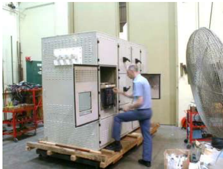
4.9 A testing engineer performing mechanical operation test.
