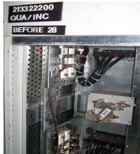
3.1.1.8 Cables and cabling accessories must be arranged to withstand short-circuit stresses and conditions
