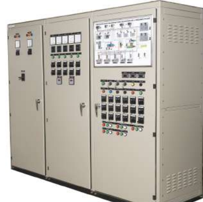
Mechanical Switchboard (Air-Con)
