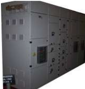
Motor control center
