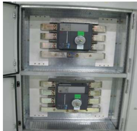
3.1.1.7a Breakers to be installed as per manufacturer's instructions, giving attention to short-circuit conditions
