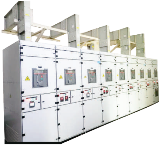
Main Switch Board
