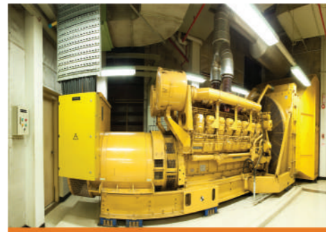
Acoustic Generator Room
