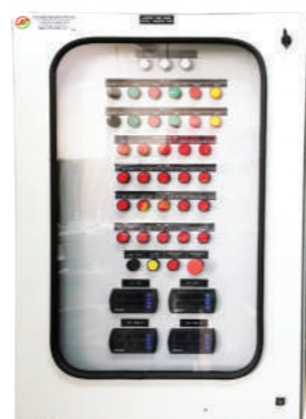
Airport Diesel Transfer Pump Panel
